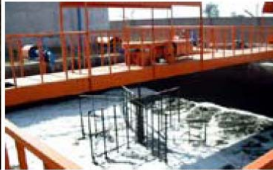
Sprinkling of EM in the equalization tank
